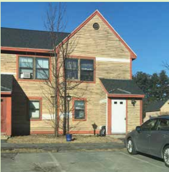
Prior to renovation, Breary Farms, above, was showing its 30 years of age, and was clearly in need of major repairs and upgrades.
